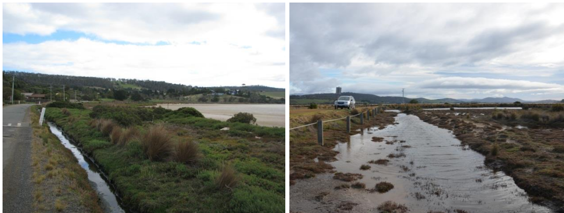
Figure 4. Left: Ditch running parallel to Bicheno Street. Right: Ditch on the southern side of Bicheno Street, by the Cape Deslacs Track, which also serves as an artificial tidal channel linked to one of the two road drainage areas.
