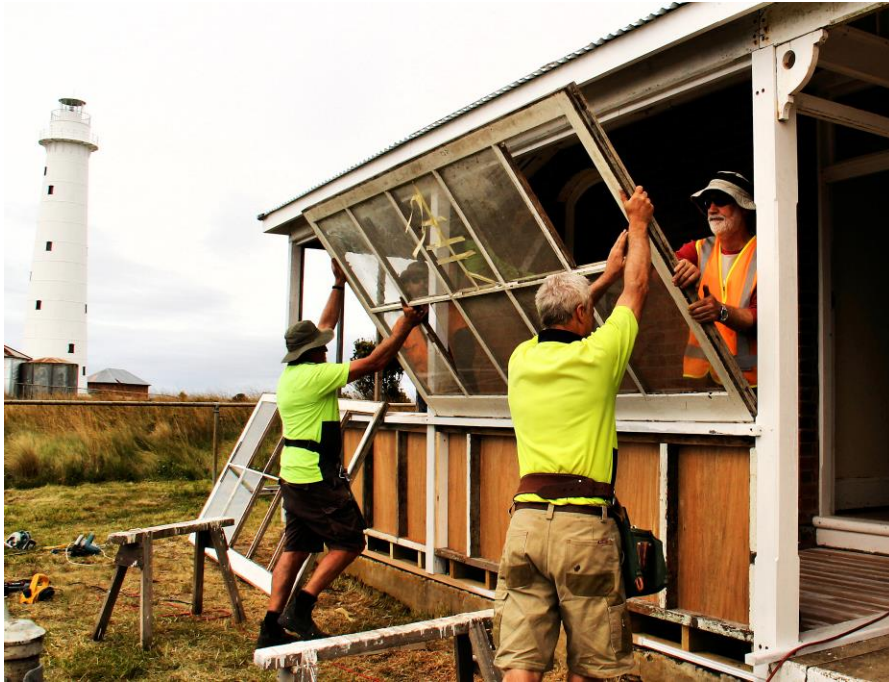
Installing the windows in the sunroom, Quarters 2: Chris Smith, Robert Banfield, Chris Creese & Mark Dickenson
