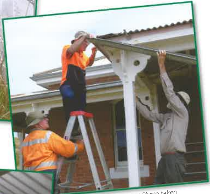
Tasman Island Gutters! Photo taken by Jan Perkins.
