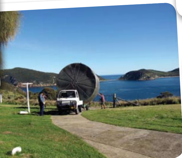
Moving the new water tank into position on Deal Island. Photo Shirley Baker
