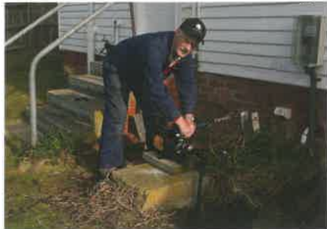
Wildcare volunteer Ron Fehlberer hard at work on replacing the pump on Cape Bruny Island lighthouse station.
