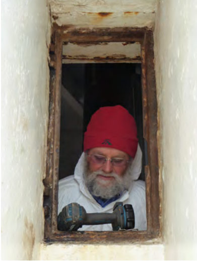
PWS volunteer caretaker working on restoration of a window in the lighthouse
