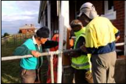
Dave scarfs some sound timber on the bottom of verandah posts at Q2. Supervised by Ron & Scott!
