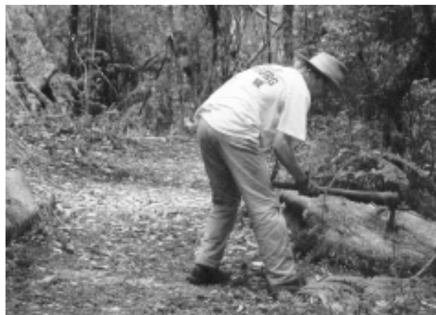
PWS Trackworker Steve Overton, carrying out maintenance work on Detention Falls track.
