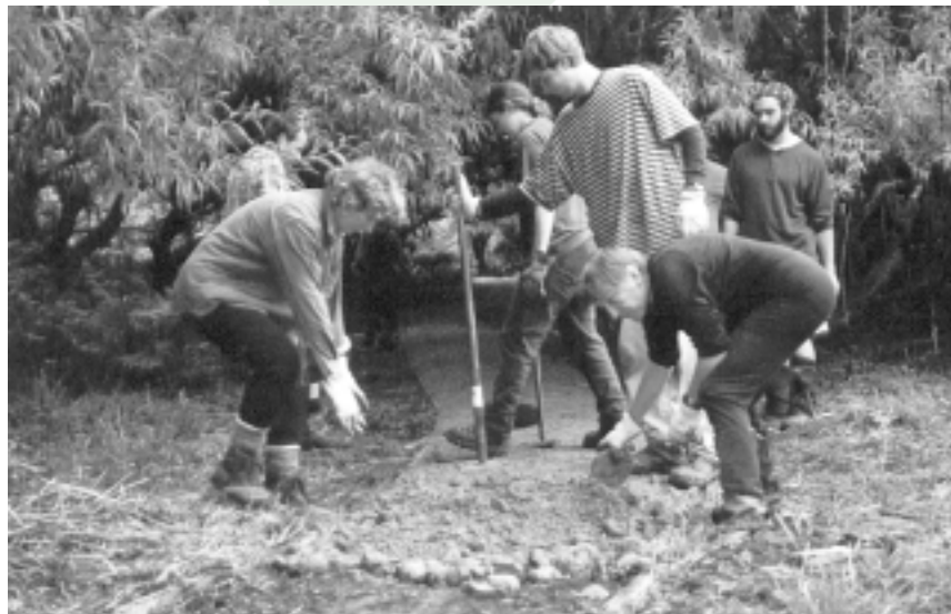
Putting in the last load on the new circuit walking track from the Oast House Ruins to Painted Cliffs, Maria Island, November 2000.
