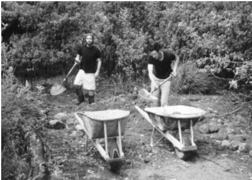
Wildcare member, Tim Baker and Alex Fichtel, USA student who has been actively involved in USA trail maintenance load up gravel for other volunteers on the Oast House Ruins — Painted Cliffs walking track.
