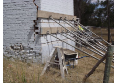
Archival picture of stabilisation of north wall of mortuary in the early days of FOBIQS
