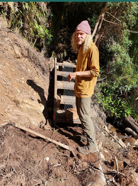
Hunter track building in landslide area, Gordon River. Photo by Sally Simco
