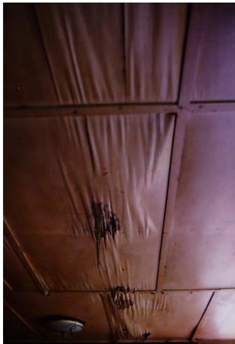
Illustration 15: Rot in ply ceiling in lounge. (Photo: D. Parham, March 2002).
