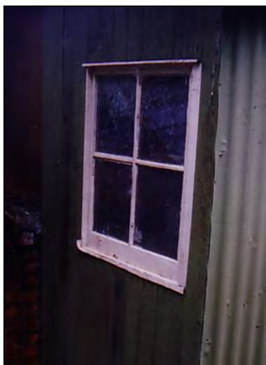
Illustration 10: Window to the laundry set in the north end of the west wall.
