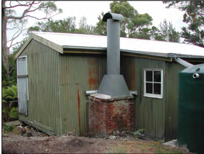
Illustration 13: View of the new flue assembly installed during PPF works in 2002. (Photo: D. Parham, February 2003).
