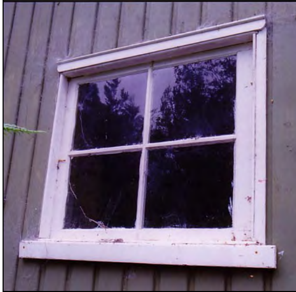
Illustration 6: Window to the kitchen south of the door in the east wall (this is W3 in Appendix 4). (Photo: D. Parham, March 2002).
