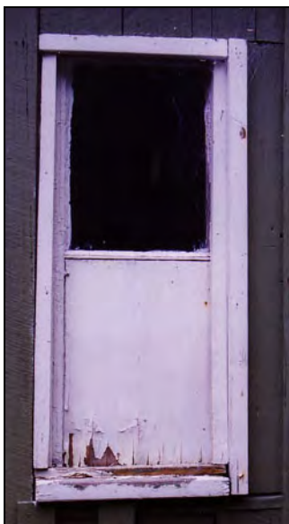
Illustration 9: Window to the bathroom in the west wall (this is W6 in Appendix 4). Note: A new window to match the original (pictured above) is being fabricated.
